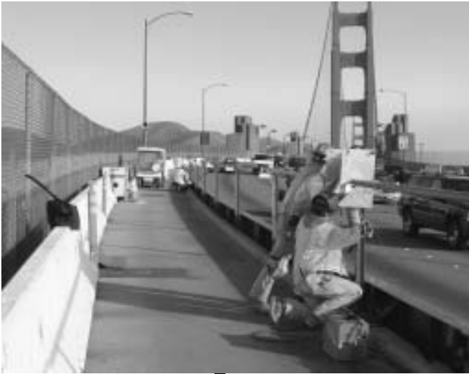
Public Safety Railing being installed on Golden Gate Bridge. Railing components were welded and painted on site.
