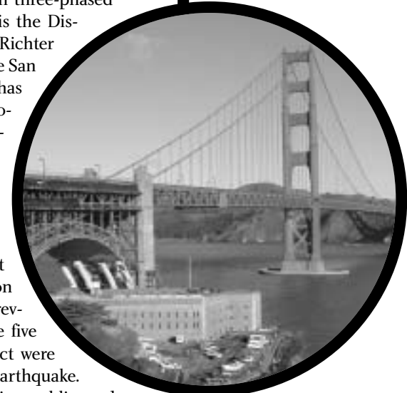
ABOVE: The most complex of the three construction phases is underway and includes the retrofit of the Fort Point arch which is situated directly over Historic Fort Point.
